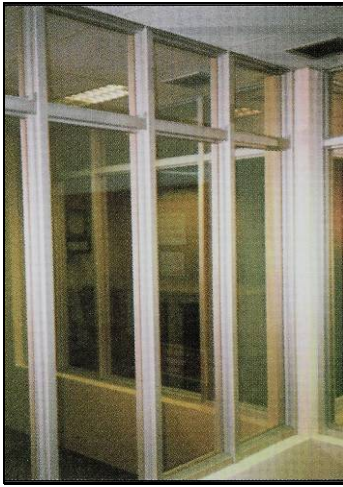
Installation of 'Datastop' in an internal screen to a control room in a water treatment plant.
