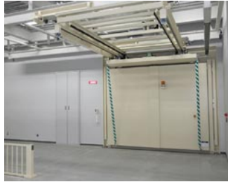
Fully shielded/closed Example of shielding door size Width: 3.6m x Height: 3m
