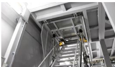
View of the stairway seen from the pit side. Safety-first electric open/close structure.
